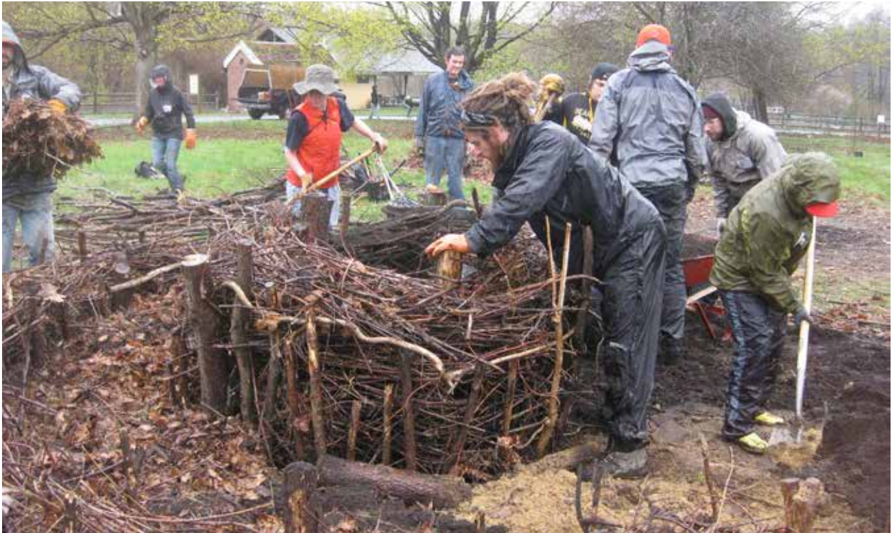
April 2014: Constructing spiral out of materials found on site and soil donated by City Soil.
